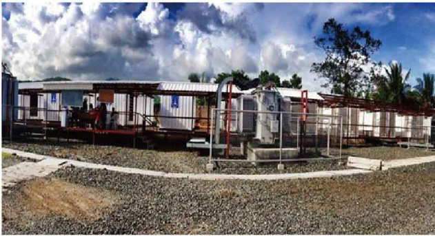
Philippines Irawan Power Plant Project
