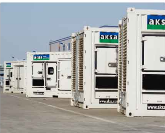
AKSA POWER GENERATION
